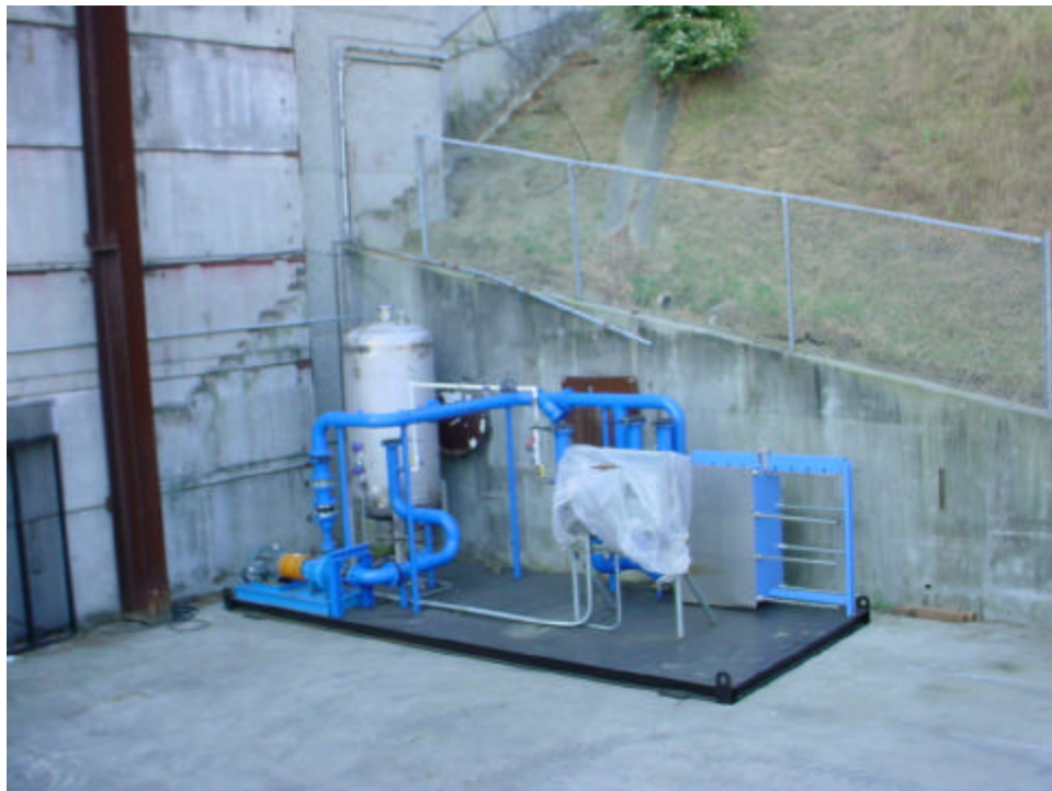
HCW pump skid in place behind B140 at SPEAR
