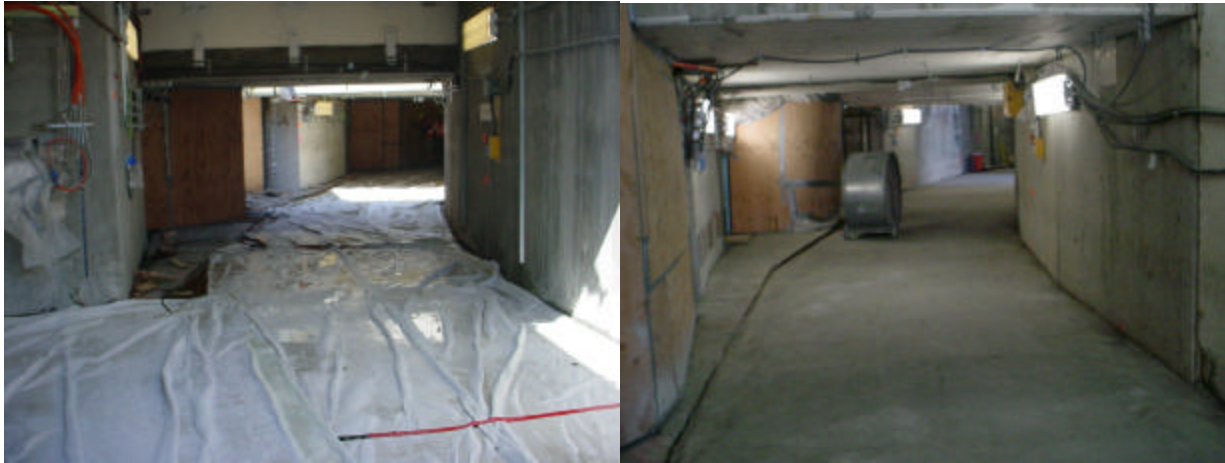
Quadrant 2 concrete curing in the left photo and uncovered in the photo at right
