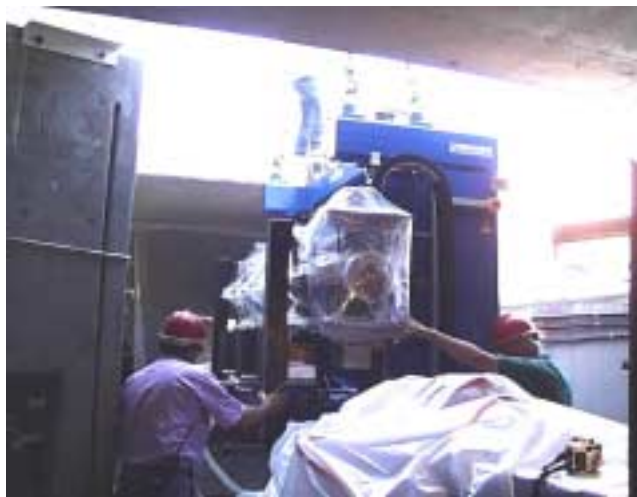
The BL11 insertion device is lowered by crane into the SPEAR ring under the careful attention of SSRL mechanical and vacuum technicians. The magnet assembly and vacuum chamber are identified as the components wrapped in plastic in the center of the photograph.
