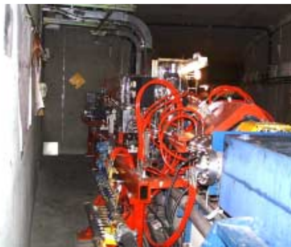
The BL11 front-end as seen at the end of the summer 1998 shutdown. The component at the lower right is a SPEAR dipole magnet. The plethora of hoses conduct cooling water to the BL11 crotch, fixed, and moveable masks as well as a SPEAR quadrupole magnet.
