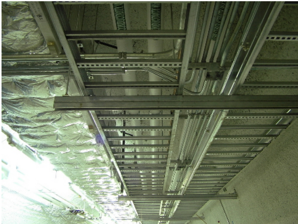
Figure 5: Ducting and cable trays
