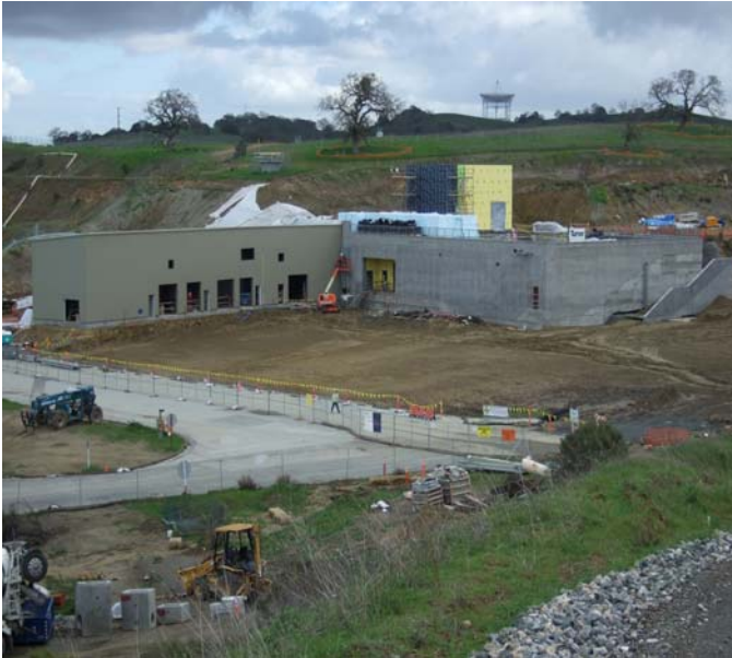
CUP and NEH with site work for Future parking lot in the forefront
