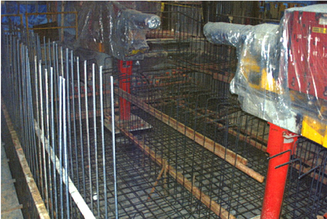
Figure 5 – Construction of new West straight section foundation and new shielding walls. SPEAR 2 magnets (under plastic cover) remain in place.
