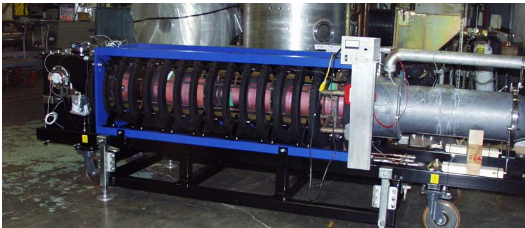
Figure 7 – The new 1.2 MW Klystron arrival
