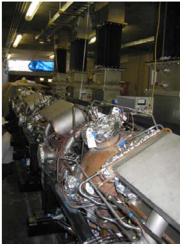
Figure 15 B - Four RF cavities installed
