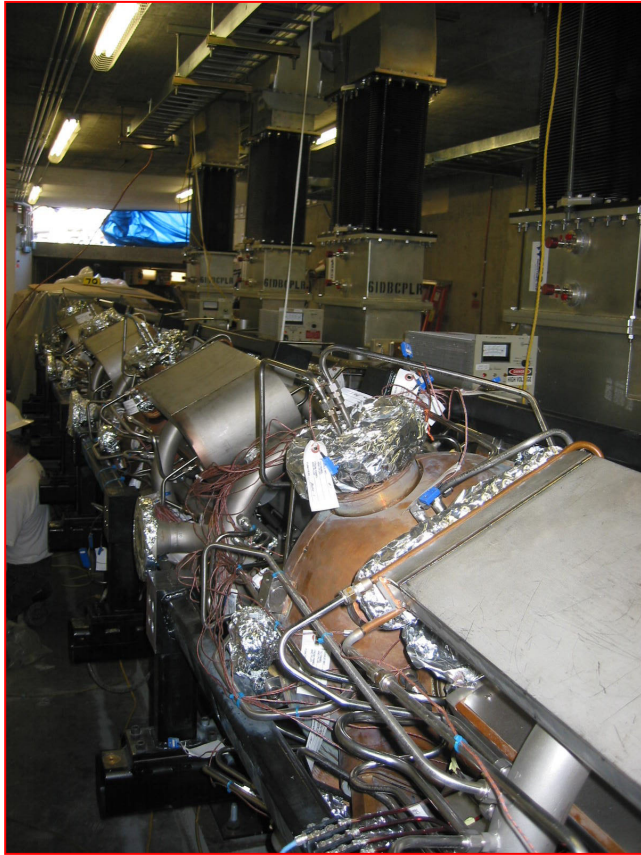
Four RF cavities installed
