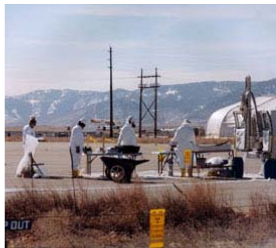
Figure 2. The 903 Pad was used in the 1950s to 1960s for storage, on bare ground, of more than 4,000 drums of plutonium-contaminated solvents and oils. The drums were removed in 1967 and 1968, and an asphalt pad was installed to control the spread of contamination.
