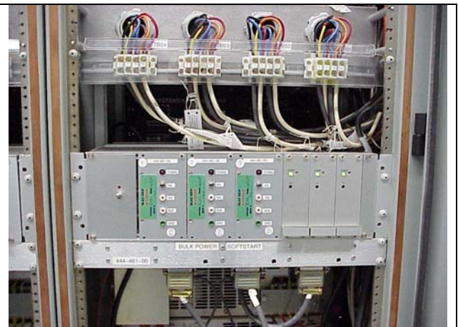
Picture 2.6b MCOR Assembly installed in existing chassis.
